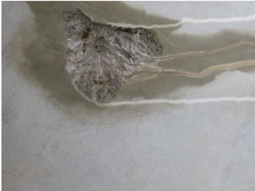
DECK PANEL BAY "D" ABUT. #1 W/ SPALL
